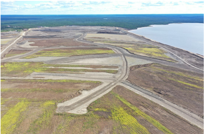
Tailings Management Area 2 - North end facing South of the Ruttan Mine Project Site
