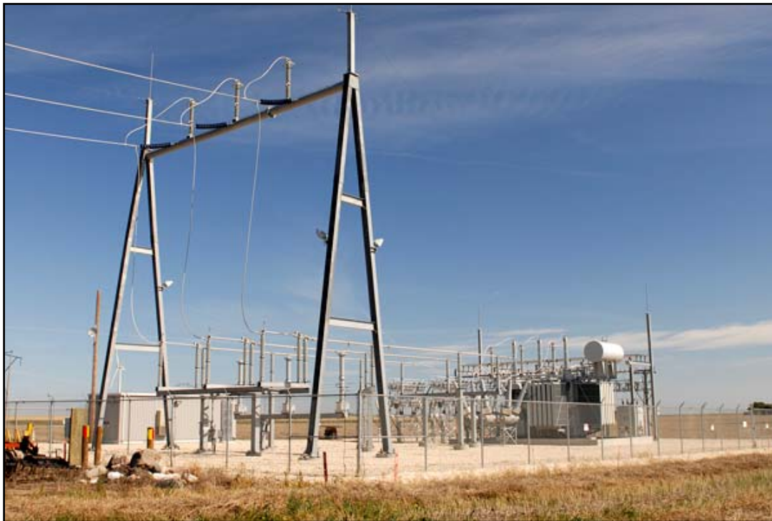
Image 6 – St. Leon Wind Farm Substation
