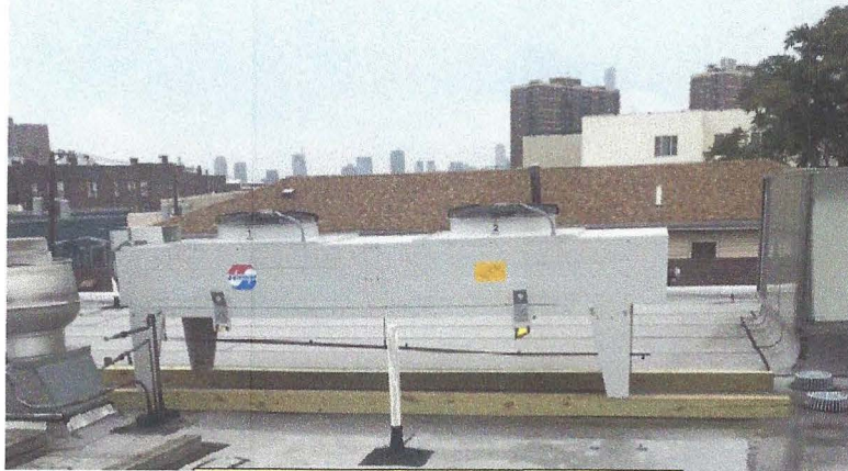
Photo example of the installed Cooler
