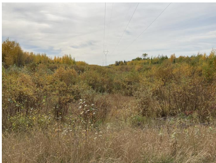
Photo 1: The Lake Winnipeg East System Improvement Project officially came in-service on June 30 th , 2018. Photo taken in September 2020.
