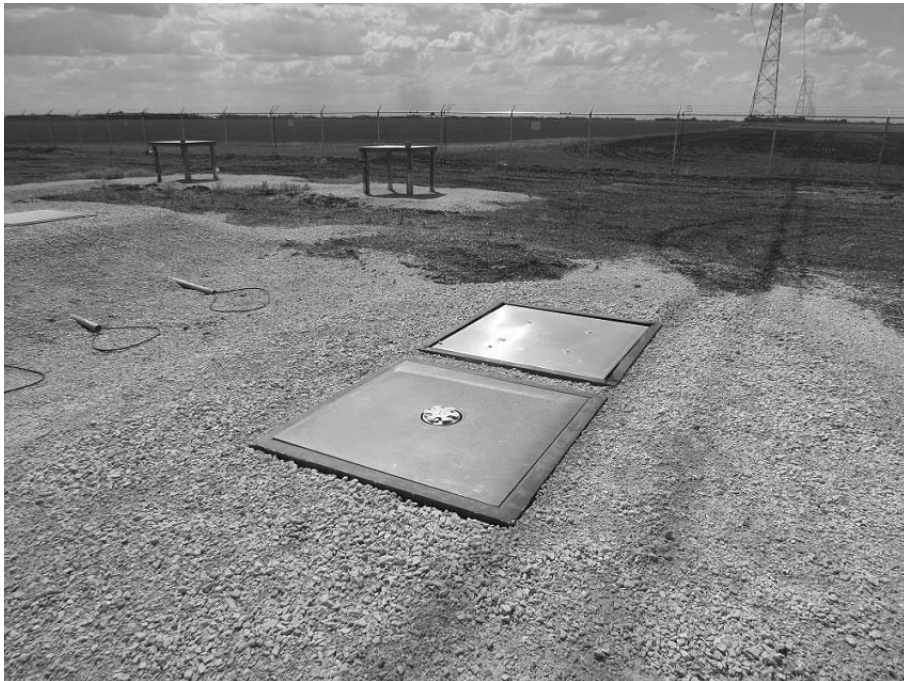
Figure 18: EFM-100 installed in center opening in ground plane metal plate over enclosure in gravel mound (in foreground).
