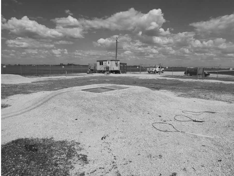
Figure 17: Main station instruments installed within enclosures in gravel mounds across the right-of-way (ROW) at mid-span.
