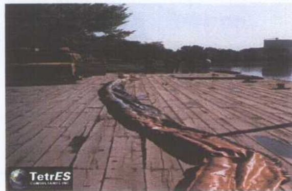
Figure 2: The boom is unrolled its full length prior to beginning the attachment of the boom mesh curtain and the mesh weights.
