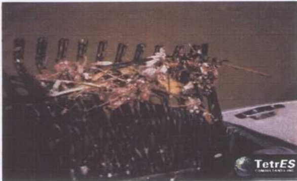
Figure 14: At the Mission outfall, one rainfall event resulted in the discharge of significant amounts of raw animal tissue. The animal tissue is seen as red material in the skimming rake pictured above.
