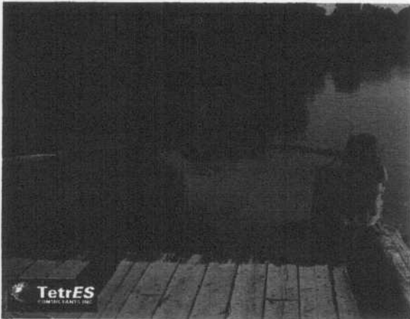
Figure 7: The Alexander CSO Boom installation involved anchoring one end of the boom to the shore and the other end of the boom to the Alexander Docks.
