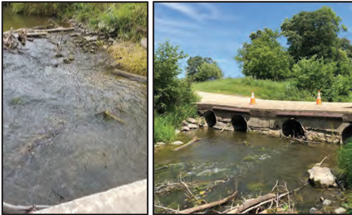
Figure 4-14 Site 6 Showing Debris Obstructions to Culvert Flow
