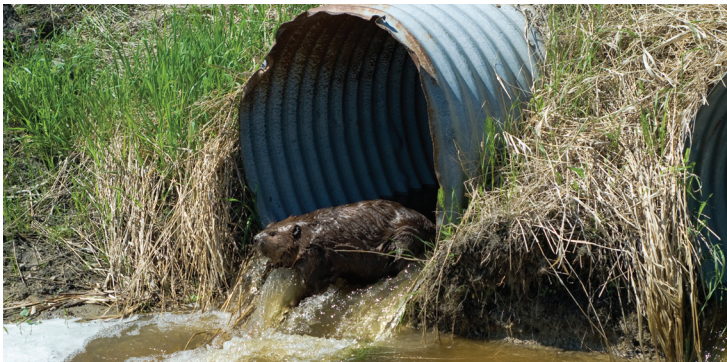
Road culverts are frequently targeted by beavers for dam construction.
