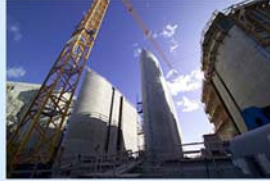
Wuskwatim's spillway will have three bays, each with a nine-metre by 16-metre vertical lift gate.
