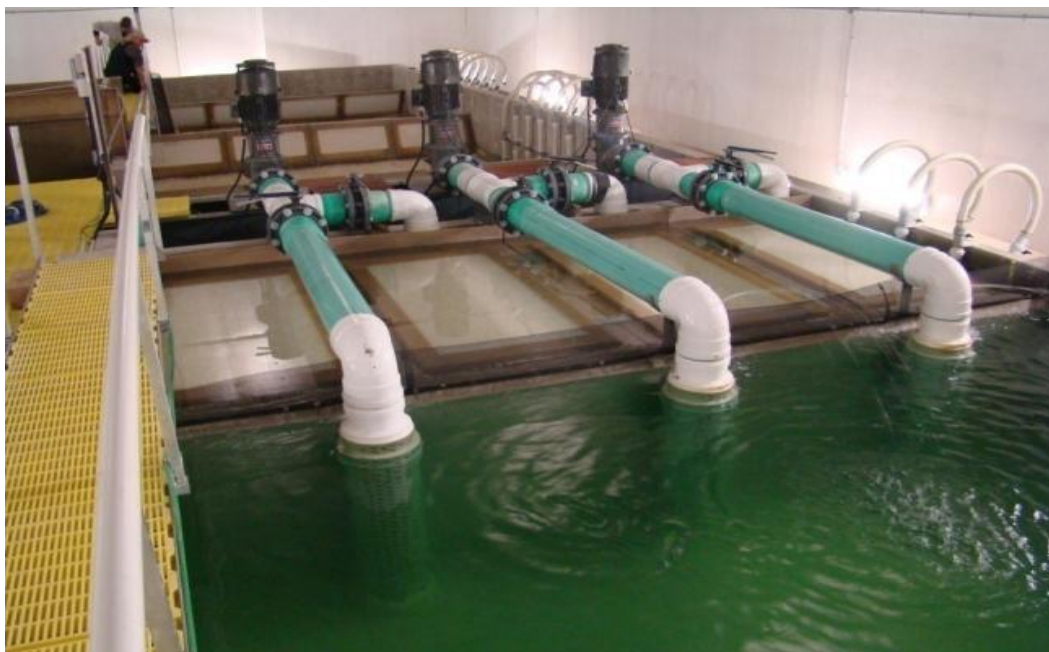
Figure 16: View of the main circulating pumps and fixed bed biofilter. Valves allow for the adjustment of flow through the fixed bed biofilter. Flow diffusers can be seen under water that help to reduce turbulence at the head of the production tank.
