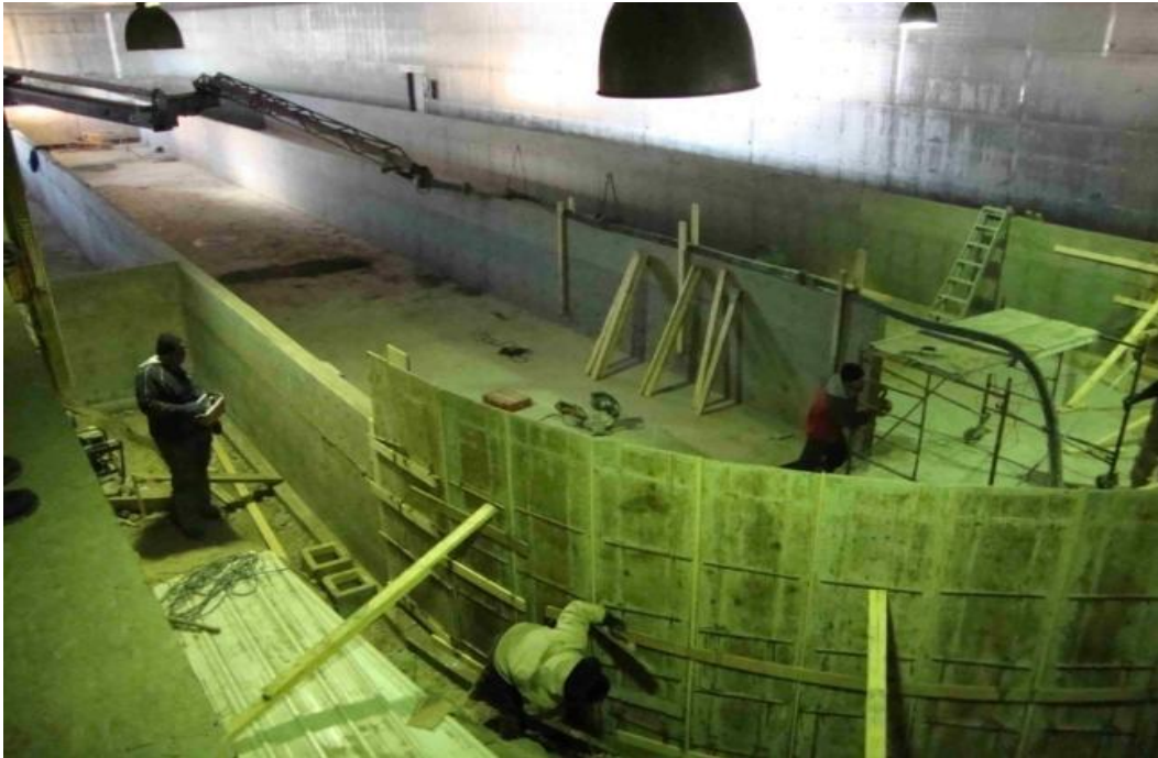
Figure 11: View of the construction crew pouring concrete into wooden forms used to construct the tank walls.
