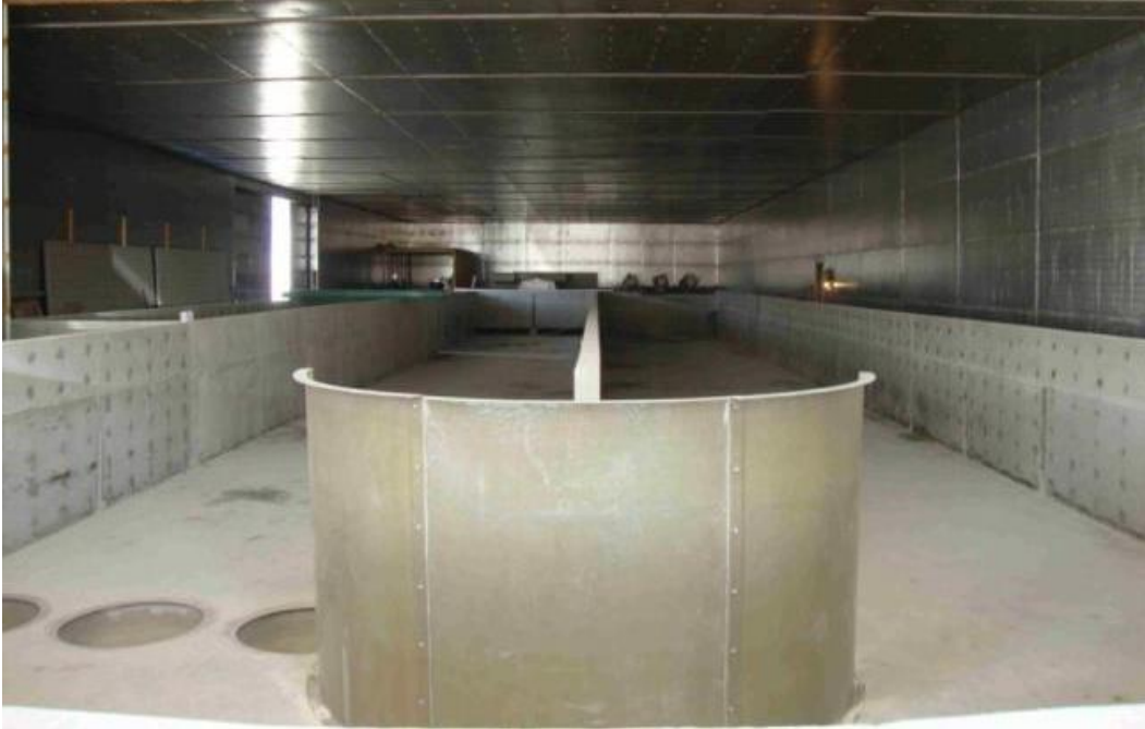
Figure 13: View of the production raceways where fish will be housed including fiberglass components such as the internal curved wall to help divert flow around the D-end as well as the upstream sludge cones that are cast into the tank floor.
