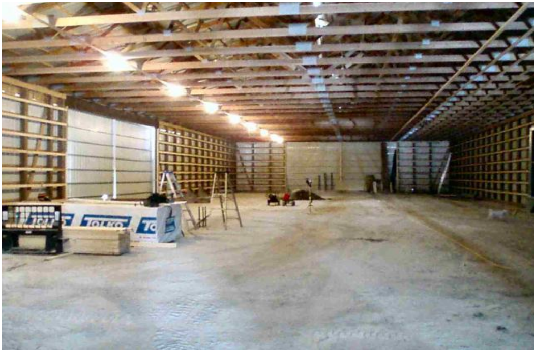
Figure 8: View of the inside of the barn being prepared for the installation of an encapsulated polystyrene insulation with reflective backing.
