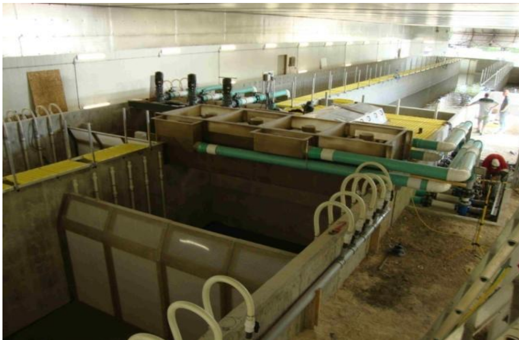
Figure 15: View of the production system with most system components installed including the over-tank walkways.
