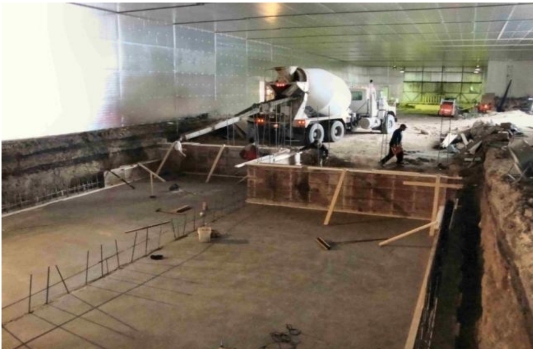
Figure 10: View of the first stage of concrete pouring. The first concrete that was poured was the floor of the water reconditioning system that sits approximately 7 feet below grade.
