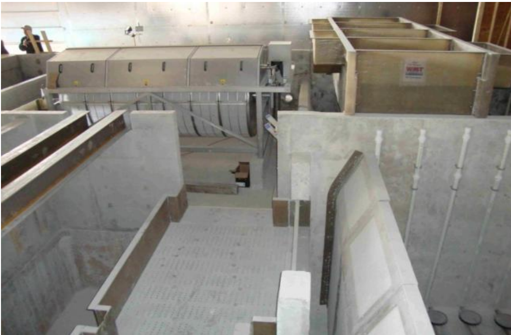
Figure 14: View of various installed components of the water reconditioning system. Namely: The LHOs, media retention screen and aeration grids in the foreground and the rotary drum filter and CO 2 strippers in the background.
