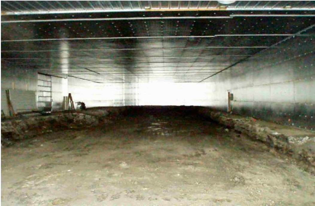
Figure 9: View of the inside of the barn following the installation of insulation and the beginning of earth floor excavation.
