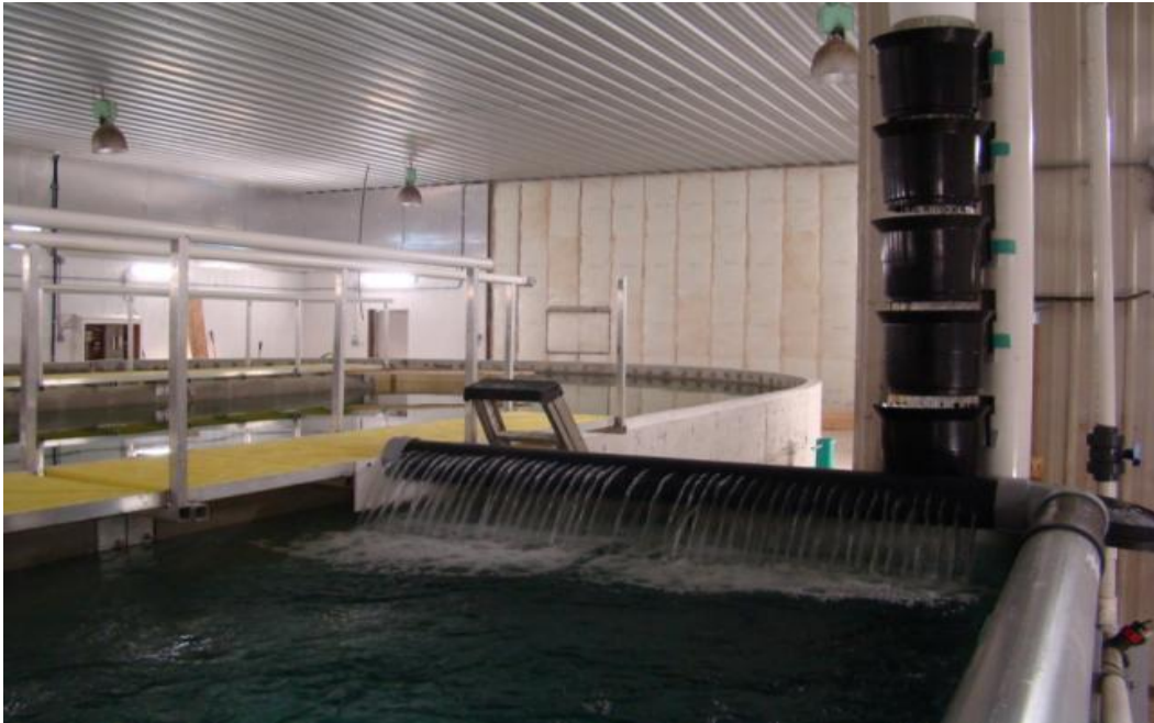
Figure 19: View of the head of the purge tank as well as the incoming well water cascading down through the degassing tower and the purge tank recirculation line below.
